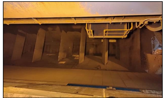
Gambar 2.3 Apron Feeder RCD 3
