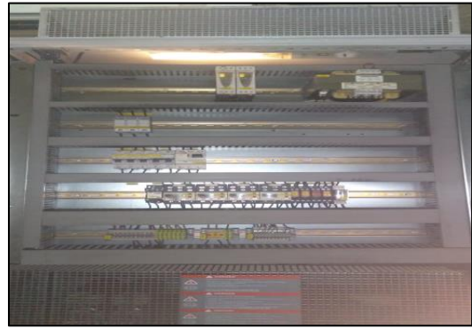
Gambar 4.1 Panel Listrik Emergency Stop Relay Trip
